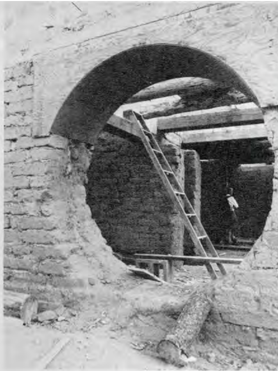
Left: View into the chapel—still to be completed when this photo was taken—from outside. The round hole was subsequently filled with Sister Giotto's Plexiglas window, seen on the first page of this article. Below: Another view of the chapel at Sagrada in progress. Bottom: Joseph's Table at Sagrada. This is the front court. Notice the adobe wall that forms a side. The small squares are tiles of the Santos and were made especially for Sagrada.
